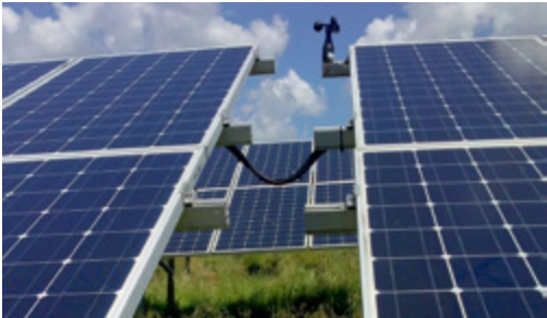
Photovoltaic power plant in Drahovce
