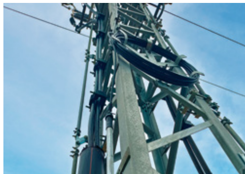
Transition of HV cable line to HV overhead line
