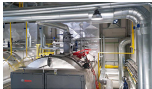
Steam boiler Bosch with accessories in the heating plant of Slovenské cukrovary Sered'
