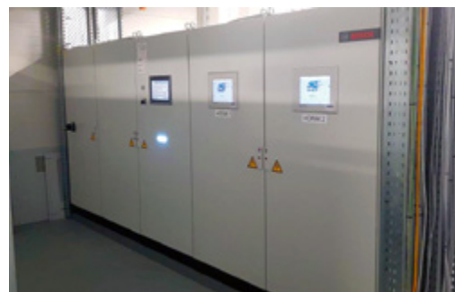
Main substation in the heating plant of Slovenské cukrovary Sered'
