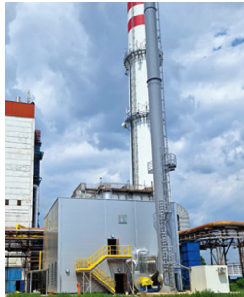
Duslo Šaľa - boiler house with new K8 boiler
