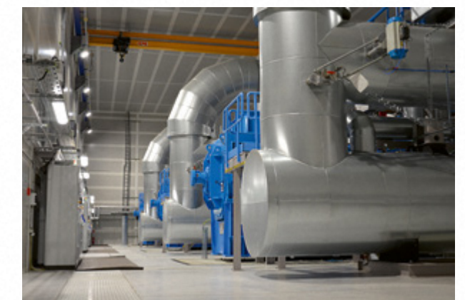
Heating plant in Martin
