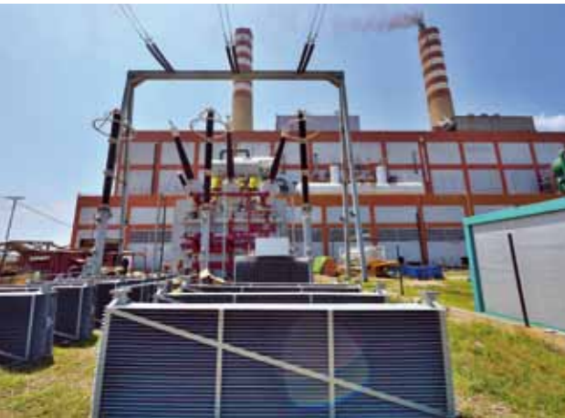
Thermal power plant in Planta Centro Venezuela
